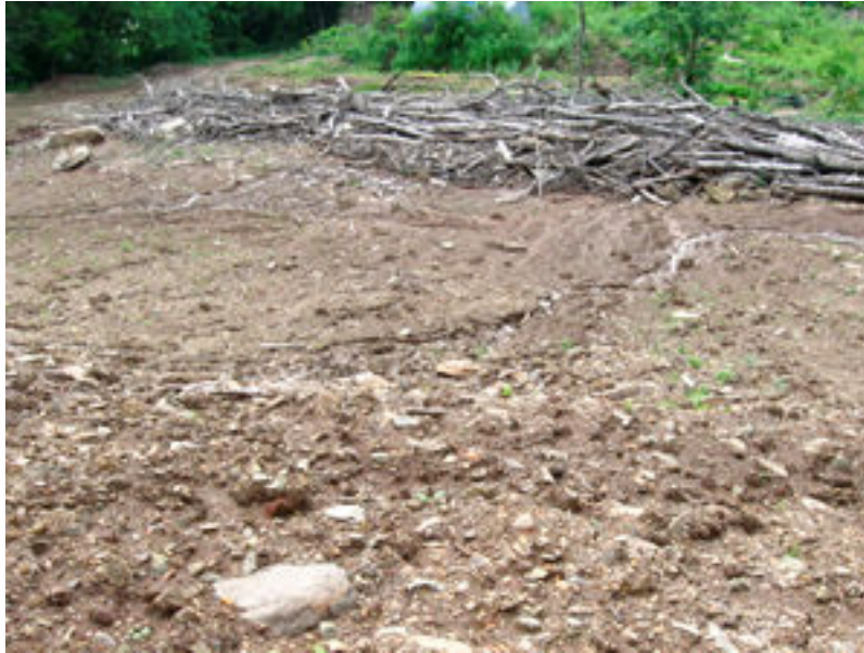
Photograph 7. This was taken looking north down the fill slope below the closed pit. Drainage erosion is visible as well as liquid drainage closer to the log pile.
