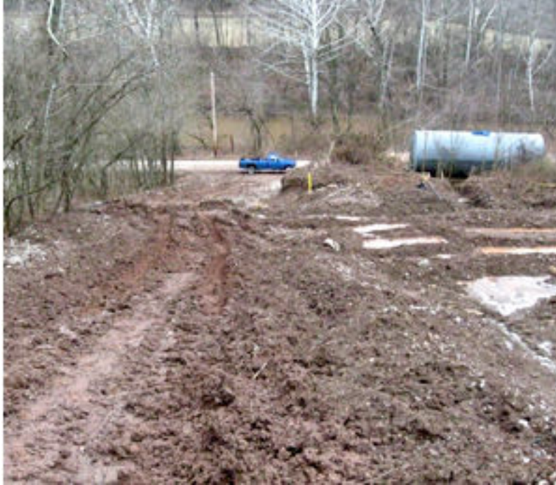
Photograph 3. This photograph was taken looking north down the well access road. The blue truck is parked by South Poca River Road and the large blue condensate storage tank is to the right. The trench through the tank's secondary containment is visible. The water bar constructed on the access road is in the middle of the photo.
