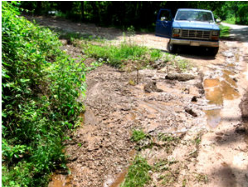
Photograph 2. The truck in the background is sitting on the well access road entrance. A culvert under the access road directs water to the western culvert. On 27 November 2008 the culvert was nearly plugged with sediment. When sediment structures were renewed in early 2009, three straw bales were placed in the sediment trap. When this photograph was taken, the sediment trap has been completely plugged and the tops of the straw bales are barely visible in the middle of the photograph. Water can be seen running in the road toward the western culvert.
