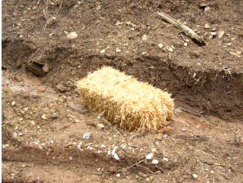
Photograph 1. Sedimentation control at this site was either lacking or insufficient. Sedimentation control structures were renewed between 12 January 2009 and 26 February 2009. This straw bale was improperly placed at this time.
