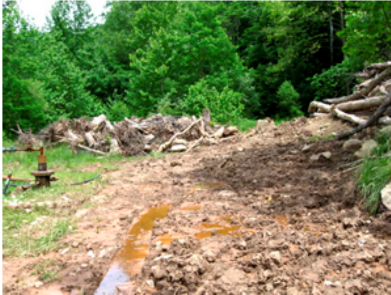
Photograph 9. This is the flat where 731 sits, looking east. The wellhead for 731 is visible to the left. The main log pile is to the right.
