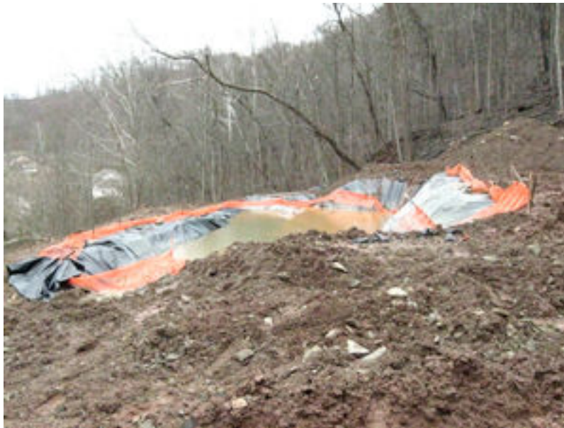
Photograph 4. This is the drilling waste pit as seen on 12 January 2009, looking east. The extent of the slip is apparent. The black material is pit liner and the orange is fallen fencing. There is almost no freeboard at the northeast corner of the pit.
