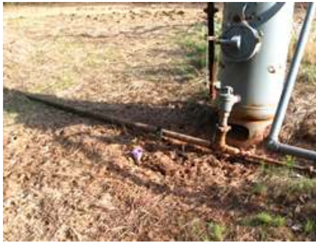
Photo 3. Pipe for oil and brine running from separator to tank (not shown). Great numbers of deer tracks along here to right up against separator.
