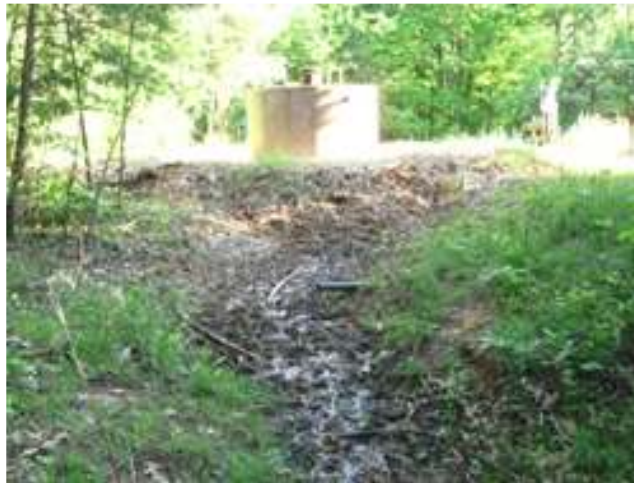
Photo 5. Ditch behind and below tank. The ditch goes a short way down hillside.
