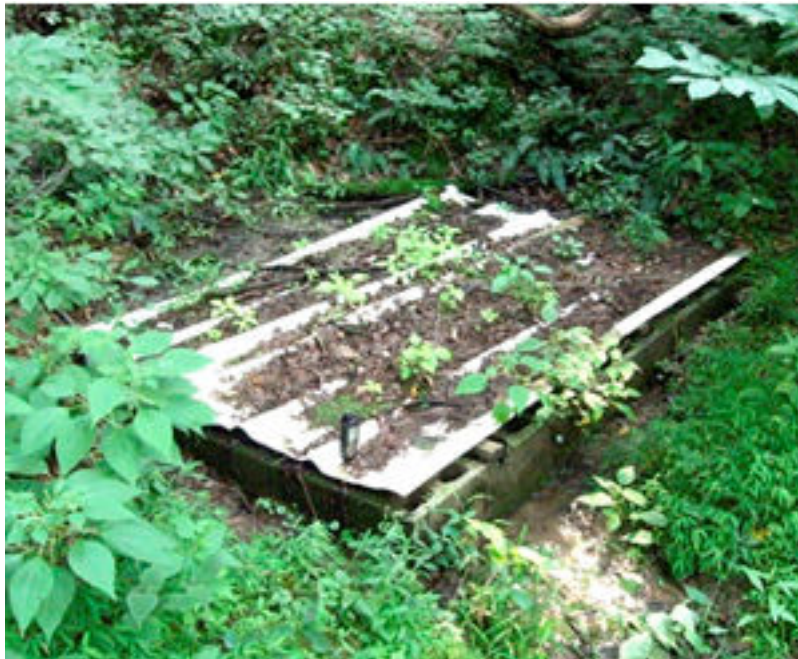
Photograph 7. The spring-fed cistern below the well pad. The cement block cistern is covered with sheets of metal roofing and its overflow drainage is visible in the foreground.
